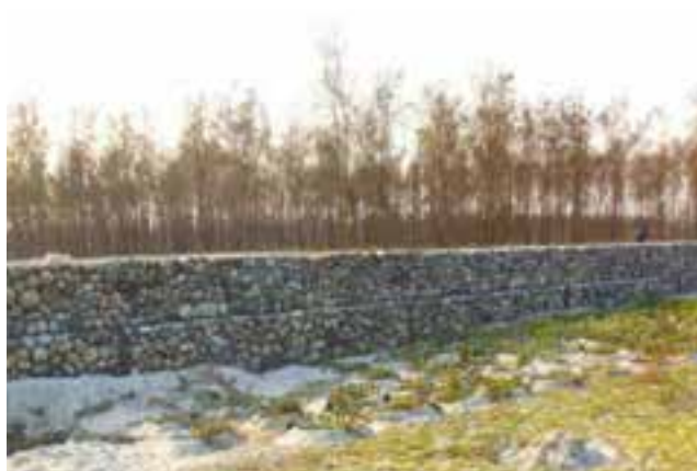
Boulder Sausage Work on Torsa River -45 mtr. at Putimari Boxirbus under Mansai Catchment Range
